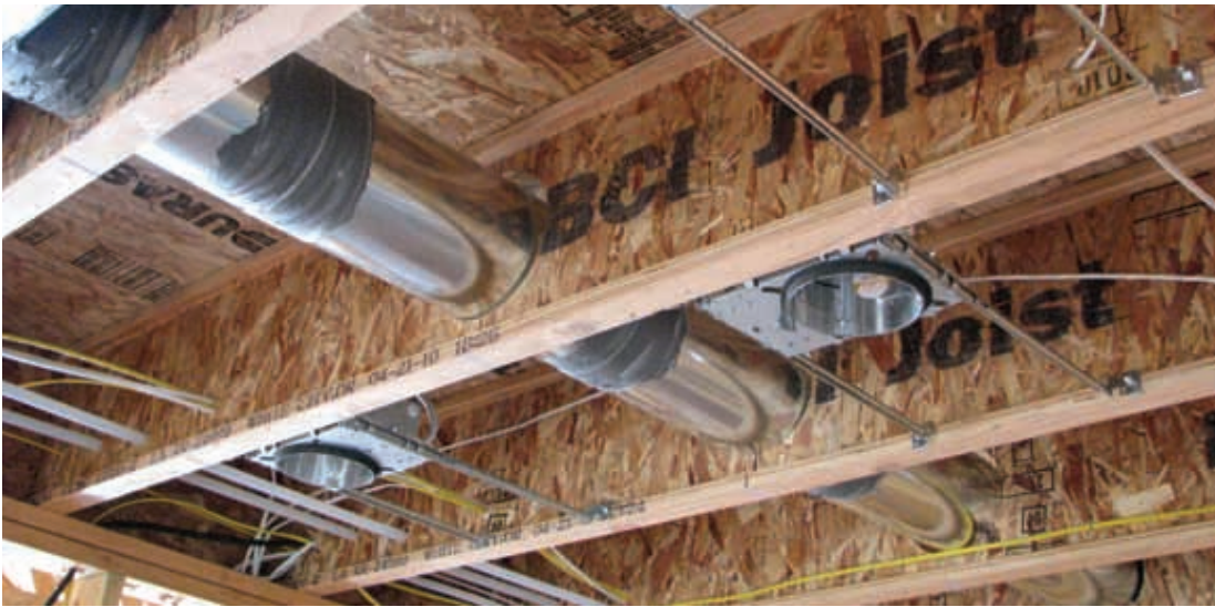
Boise Cascade Conditioned Air HVAC framing system installation summer 2010 in Central Point, Oregon by Vision Homes of Medford, Oregon. HVAC work by Spring Air Heating & Cooling, Inc. of Jacksonville, Oregon
