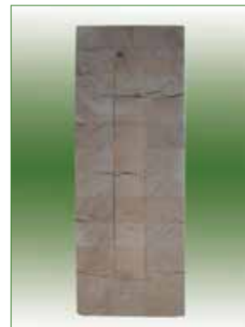
Example of Checking
