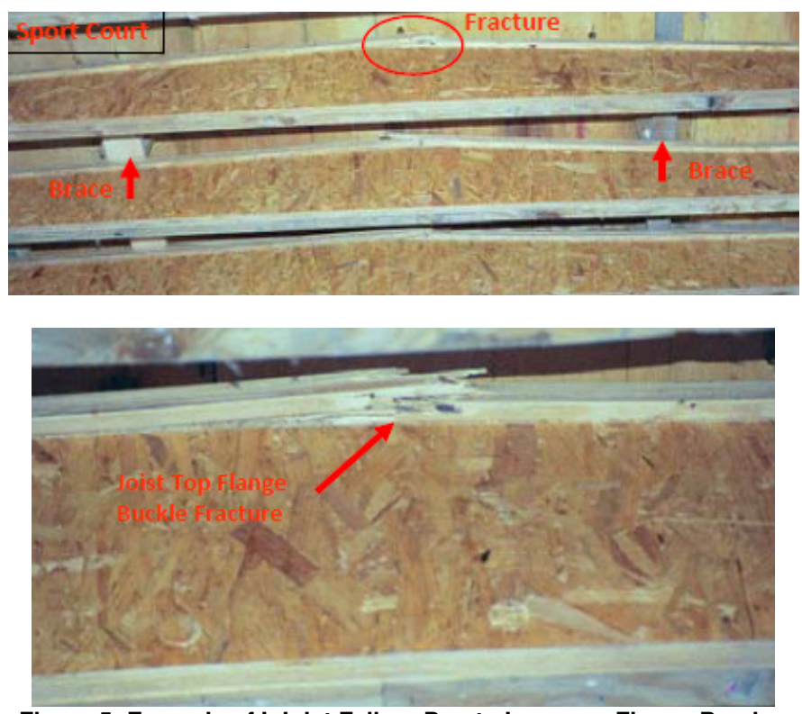
Figure 5: Example of I-Joist Failure Due to Improper Flange Bracing
